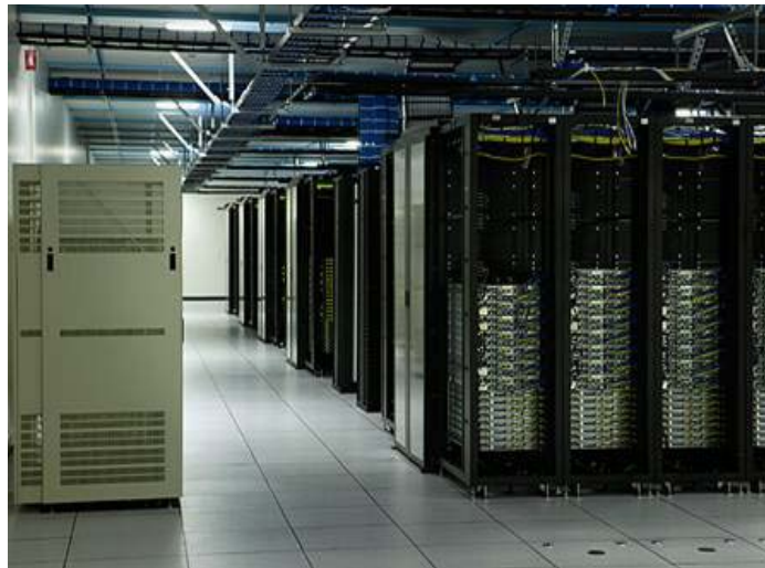
Fig 3: Typical Server room
