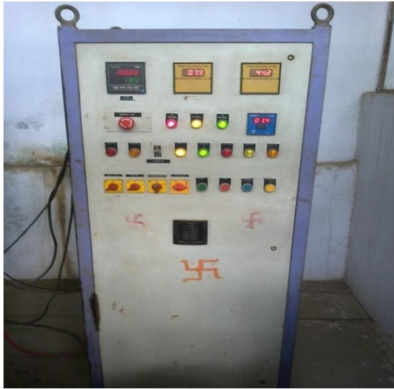
Figure :3 control panel
